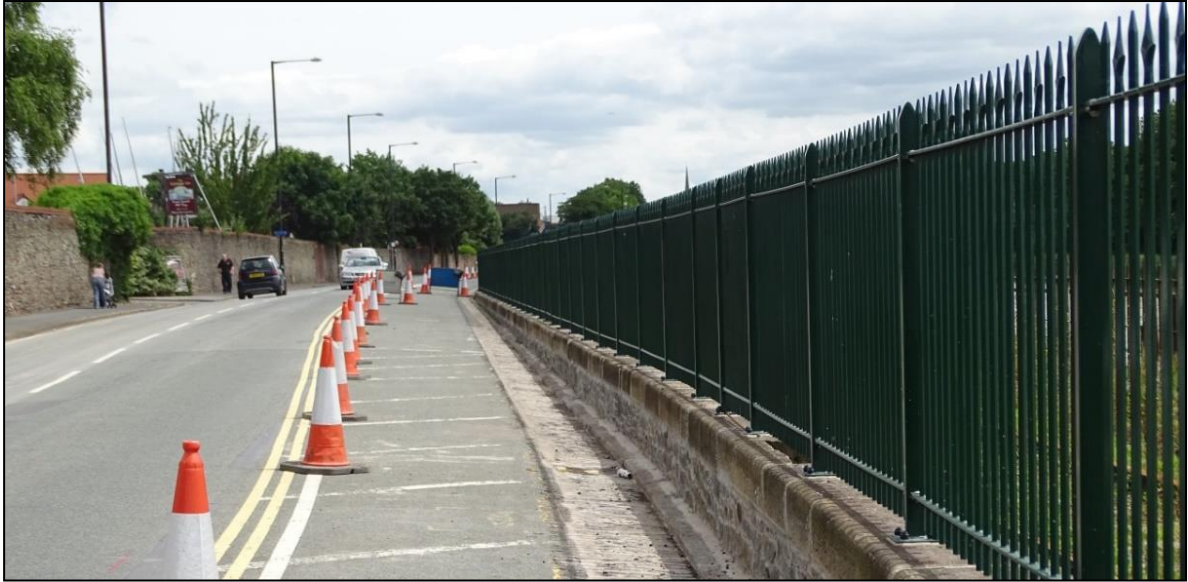
Figure 17 - The MetroBus flood wall on Cumberland Road
